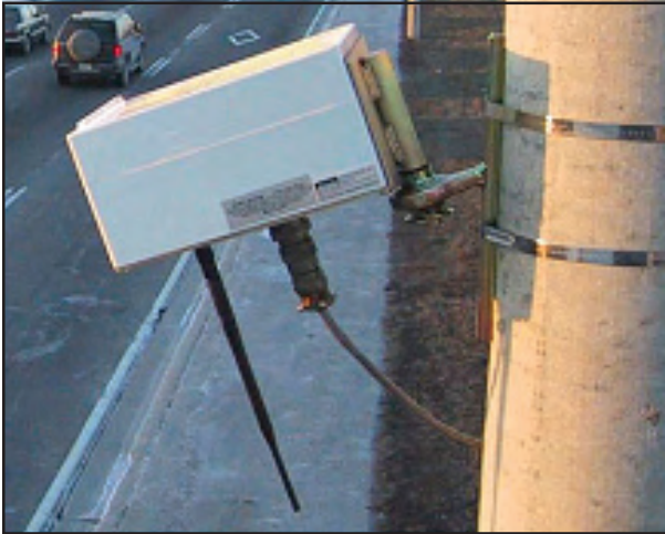
Figure 5 – Microwave Detection Unit (Side-Fire Mode)
