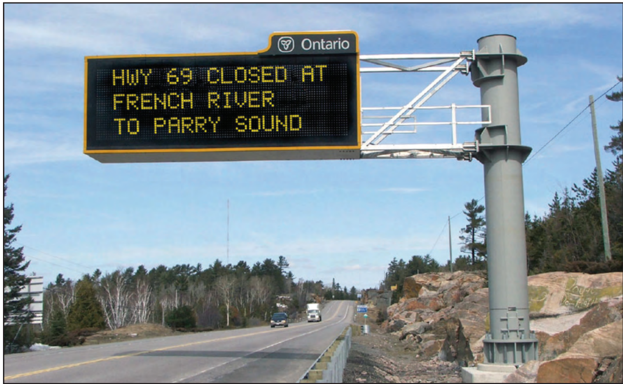
Figure 13 – MTO Roadside-Mounted (Cantilever) DMS
