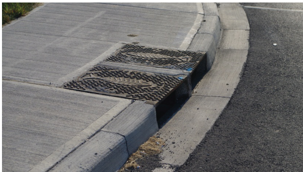
Figure 5.46 – Catch Basin Inlet within the Curb Face
