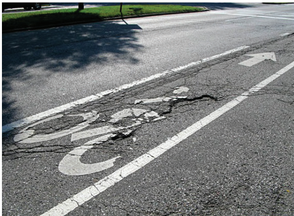
Figure 8.2 – Poorly Maintained Bicycle Lane
