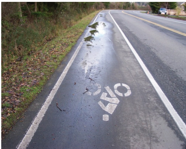
Figure 8.5 – Poor Drainage Causes Puddling in Bike Lane
